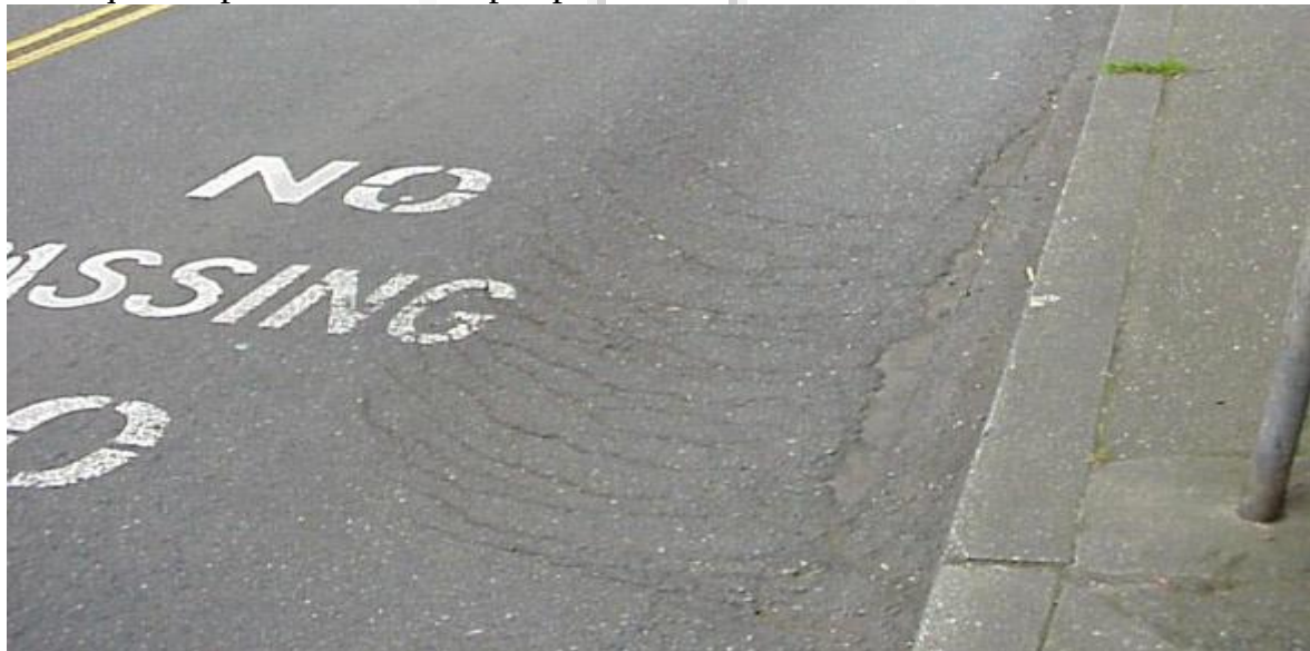
Fig. Slippage Cracks
