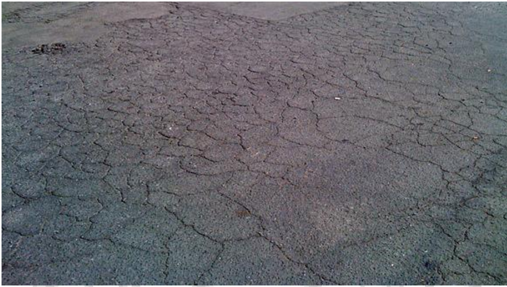
Fig. Alligator Cracking
