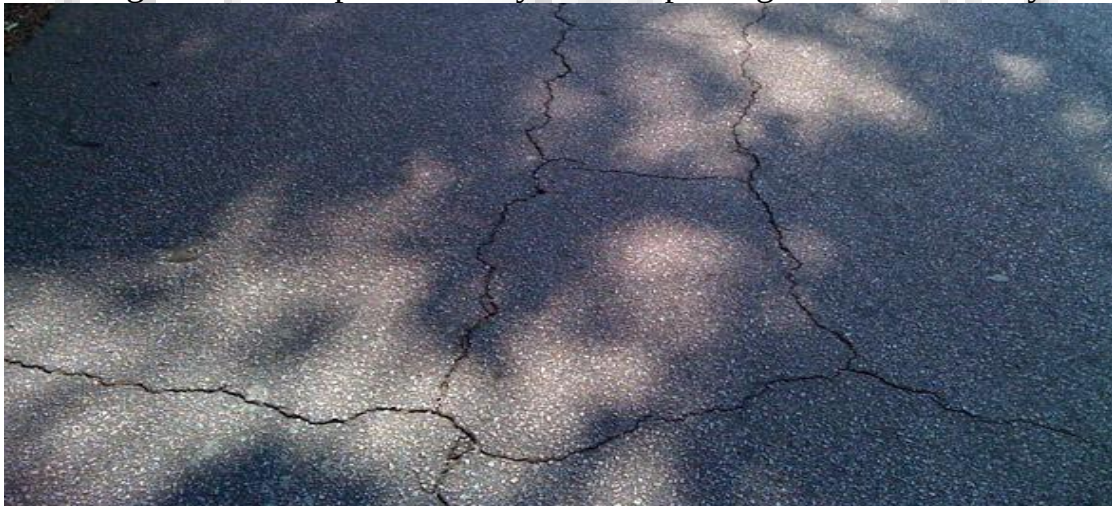
Fig. Block Cracking
