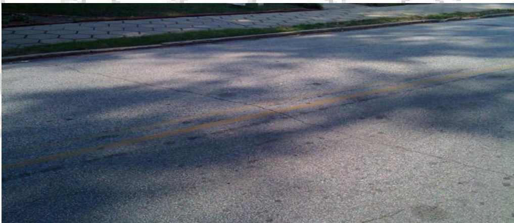
Fig. Transverse Cracking
