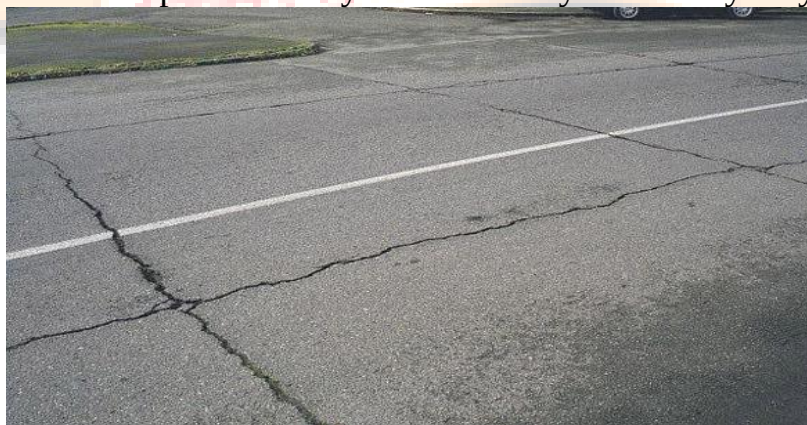
Fig. Joint Reflection Cracks
