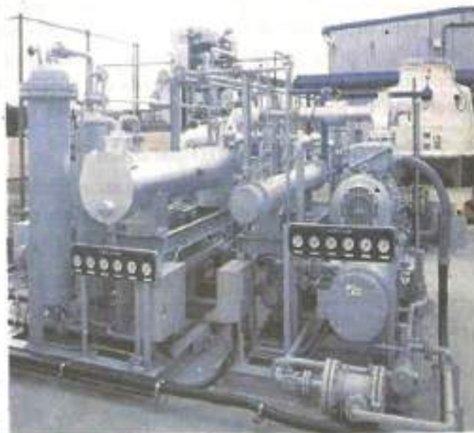
Ultra-low temp. refrigeration system using \text{CO}_2 and \text{NH}_3 for industrial applications.
