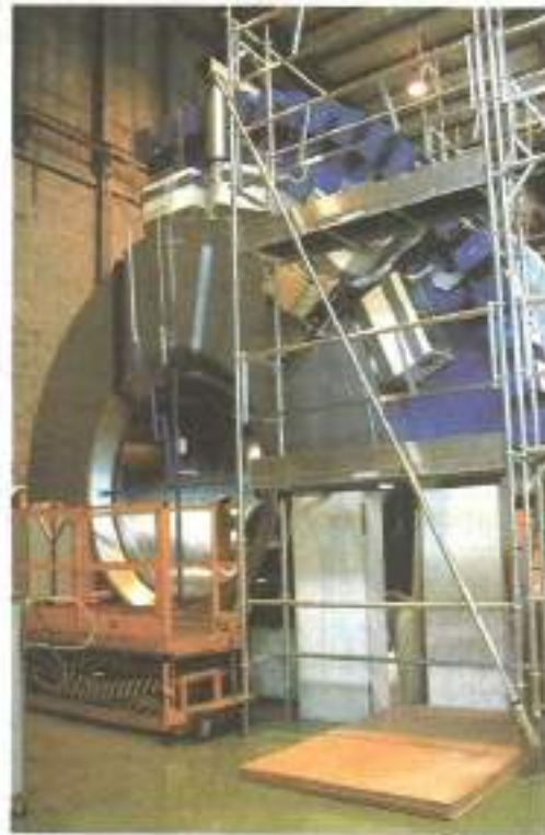
Air evaporative cooling system
